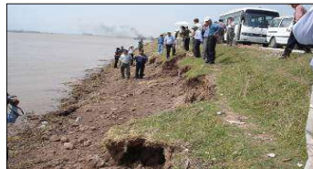
650m sea dyke without mangroves at Thái Đô was partly destroyed in the Storm No. 2 in 2005
