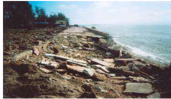
Without mangroves protection seadyke in Cat Hai was destroyed Storm No 2 in 2007
